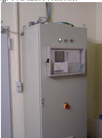
Fig. 2 AMESA control cabinet
